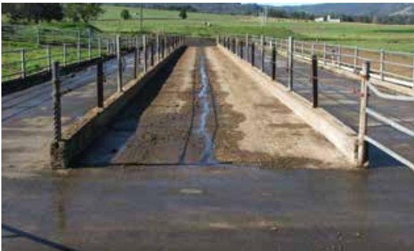
PMR fed out on fully concreted feedpad with nib wall, central feed alley
