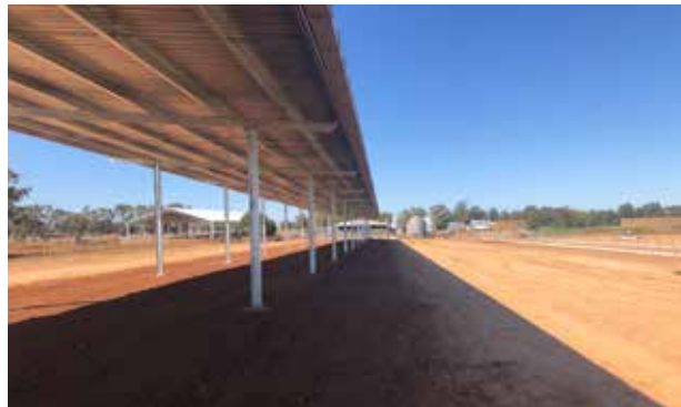
Stand alone cattle shelter with spouting and downpipes to remove rainfall
