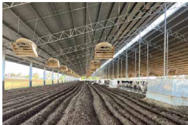
Figure 42. Mechanical ventilation (fans) – fans hung high enough to avoid equipment operating in bedding area
