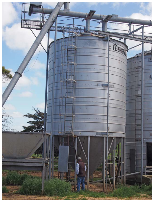
Silos showing caged ladders and sight glasses.
