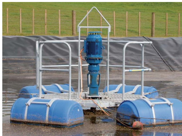
Well-constructed stable pontoon with lifting point. Source: DairyNZ Farm Dairy Effluent Systems
