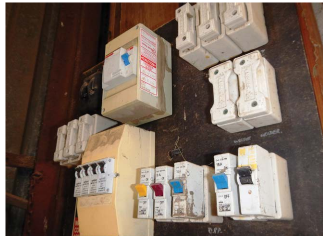
RCD on switch board is tested and tagged.
